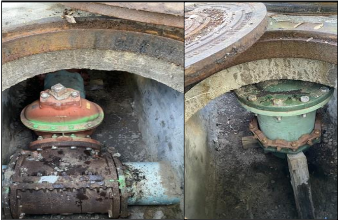
Pig Launching Structure At lift Station 39 SAVANNAH savannahga.gov
