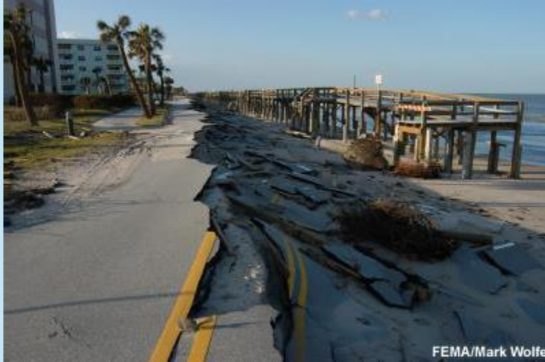
Beachfront road and boardwalk damaged by Hurricane Jeanne (2004)
