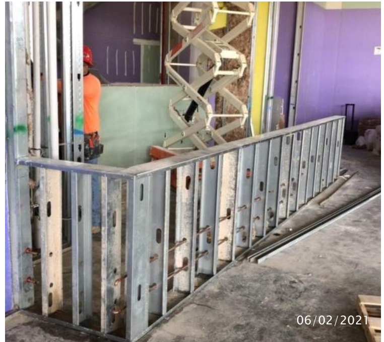
Concourse Quad 2 - Crews framing knee walls at North Club Bar - Looking Northeast.
