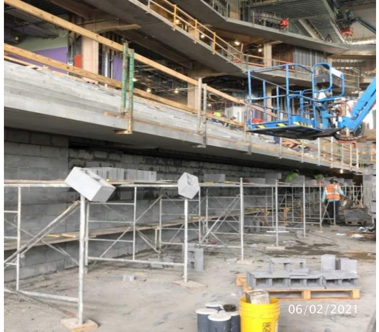
Event Level - Crews continue masonry under precast rakers in Quad 2 - Looking Northeast.
